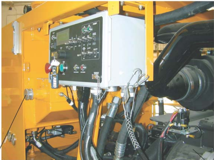
CONTROL BOX WITH COVER REMOVED
