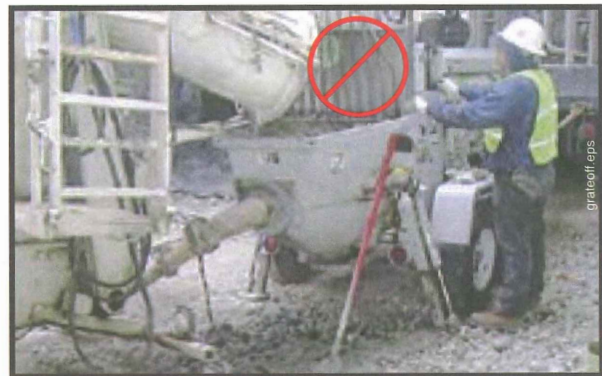
Figure 26 Never remove the hopper grate while the pump is operating
